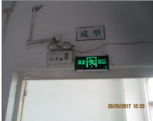
Photo of fire safety equipment Exit sign and emergency light.JPG
