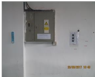
Photo of the inside of the main production hall Electricity control box with warning sign.JPG
