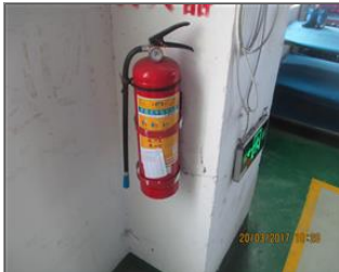
Photo of fire safety equipment Fire extinguisher.JPG
