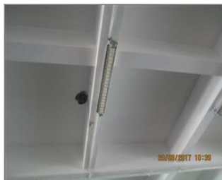
Photo of the inside of the main production hall Explosive-proof light.JPG
