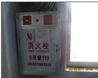
Photo of fire safety equipment Fire hydrant.JPG
