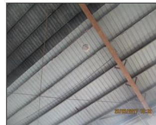
Photo of the inside of the main production hall Smoke detector.JPG
