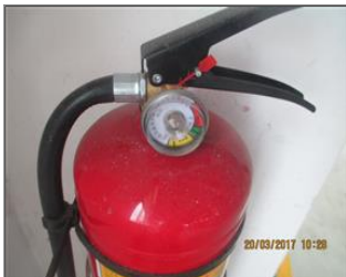
Photo of fire safety equipment Fire extinguisher with proper pressure.JPG
